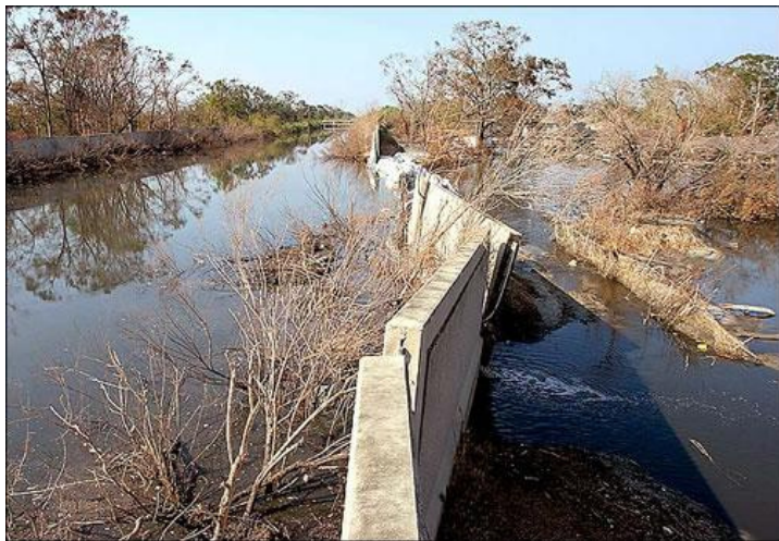
Flood protection equipment in New Orleans after passage of hurricane Katrina
